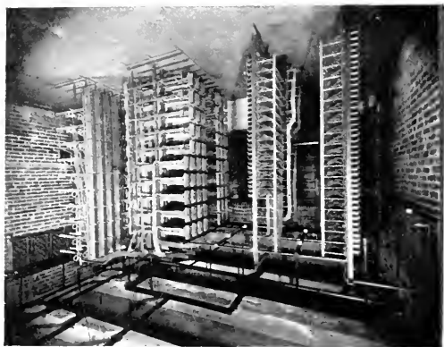
FIG. 9.—MAIN AND INTERMEDIATE DISTRIBUTING AND RELAY RACKS, EAST BRANCH EXCHANGE.
